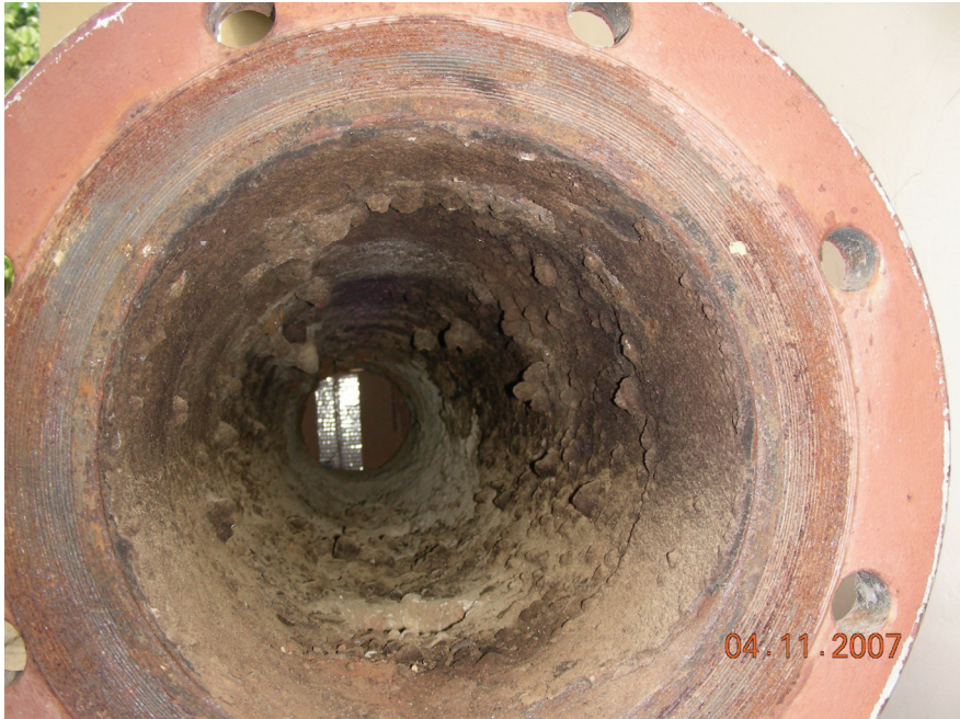
Figure 2. Photography showing the fouling layer formed in a duct section that transports crude oil (Petrobras-BR)
